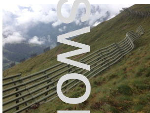
Fig. 9: example of damages to the crossbeams in the structure of snow bridges
