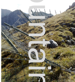
Fig. 8: example of damages to the structure of snow nets
