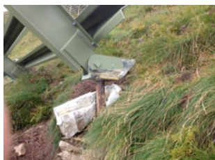
Fig. 6: example of the failure of the foundation plinth on the support of a snow bridge
